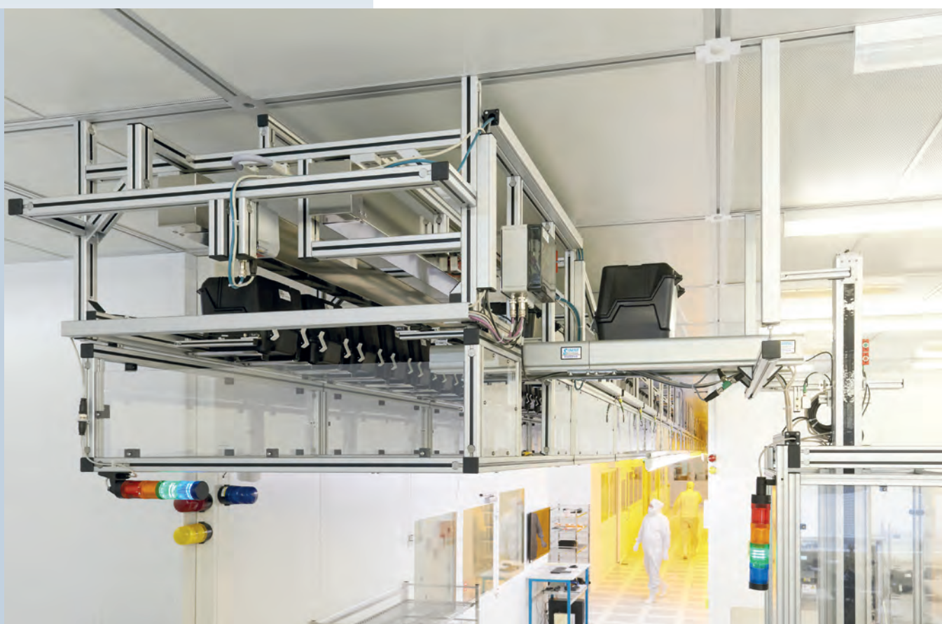
FlatStocker installation with 200 storage bins at Fraunhofer IPMS Dresden, Germany
